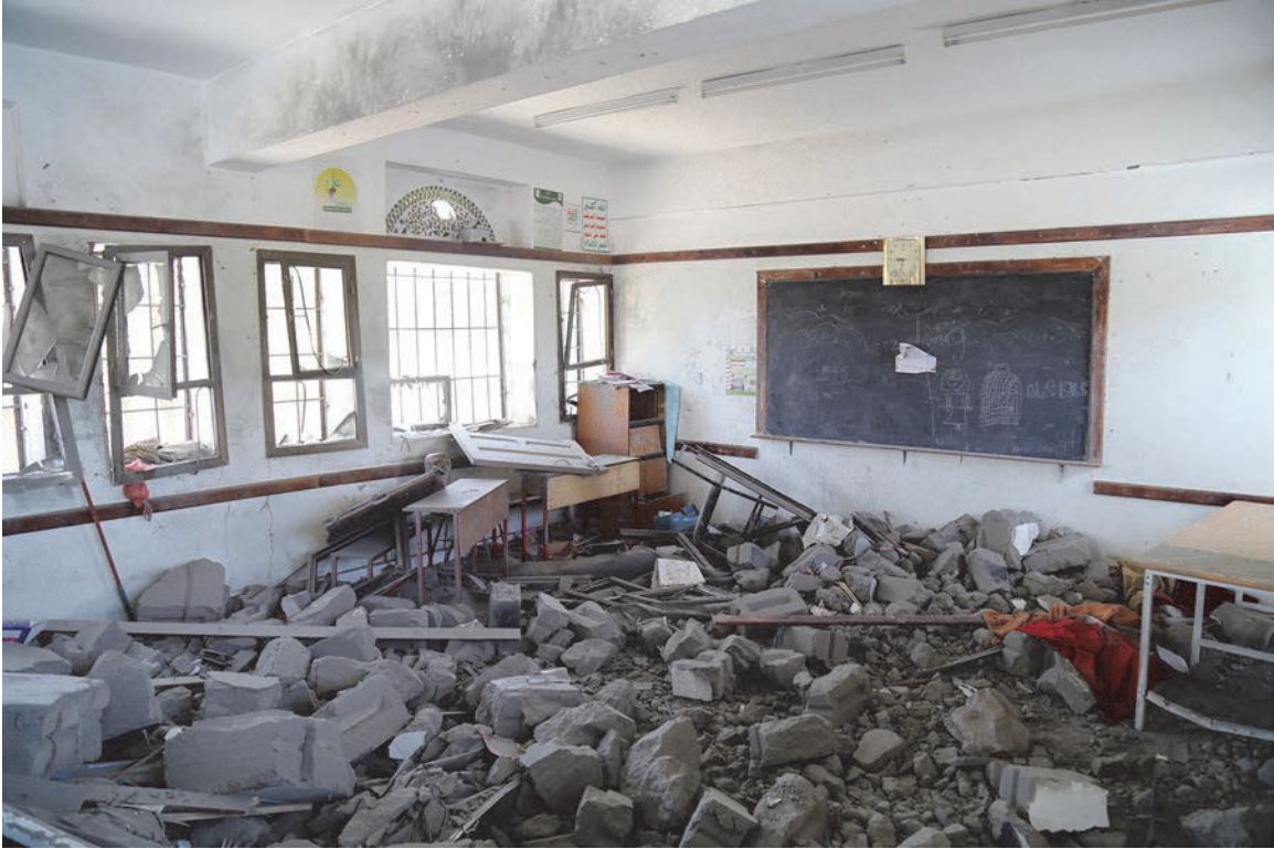
A damaged classroom in the al-Munadil Hussein Fayed School, which was struck by an aerial attack on May 11, 2015. © 2015 Ole Solvang/Human Rights Watch
