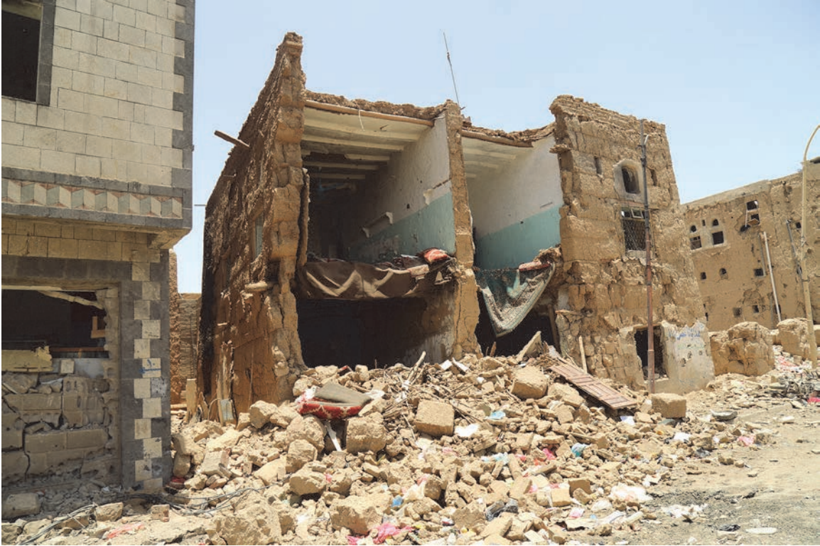
The remains of al-Sherif's house, which was hit by an aerial attack on May 10, 2015, killing at least four civilians. © 2015 Ole Solvang/Human Rights Watch
